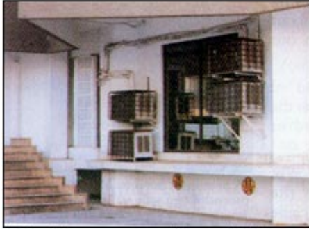
The side entrance to a well known building at Nariman Point. Notice the standard cages around the ACs and the exposed refrigerant piping. Not so nice to look at !
