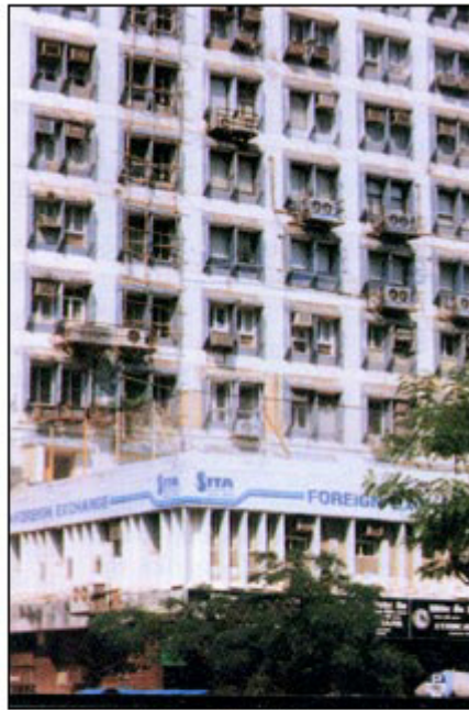
Another landmark building at Nariman Point whose facade is plastered with ACs and service enclosures. Other buildings have soft PVC piping carrying condensate and looking like spaghetti stuck on the facade.
