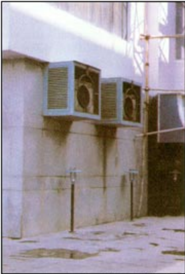
A prominent hotel on Marine Drive has concealed two split AC "outdoor" units to improve their appearance and reduce the effect of sea air corrosion
