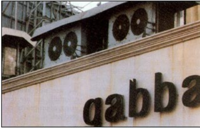
Prominent retail stores on Warden Road have built ugly cages and rain/sun shades over their split AC units
