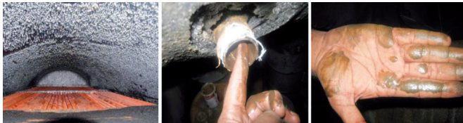
Figure 2: Corrosion of cooler shell due to water
