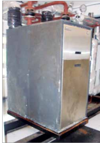
Heat Pump in plant room
