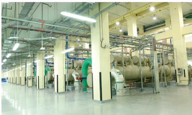
Photo 11: Service space around chillers
