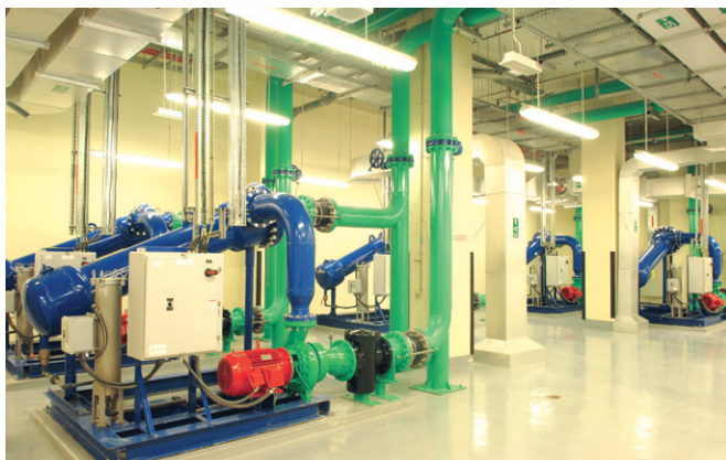
Photo 8: Independent filtration unit for individual cooling tower cells
