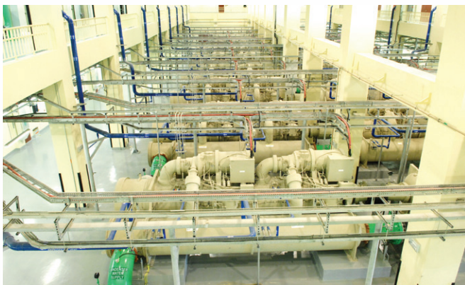
Photo 2: View from mezzanine floor balcony – battery of chiller modules
