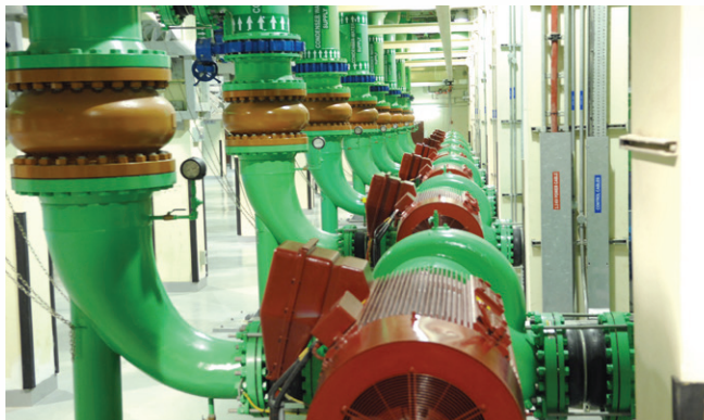
Photo 10: Cooling water pump installation with NRVs, discharge volutes and flexible connections
