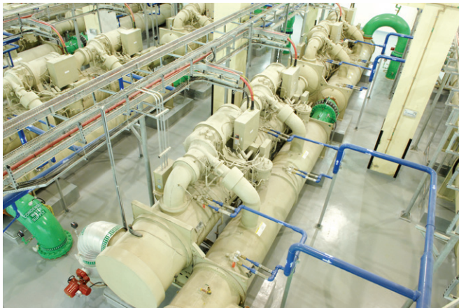
Photo 1: Evaporator and condenser water pipe connections
