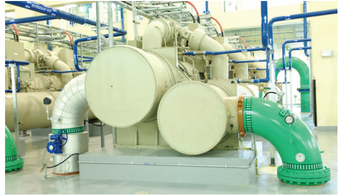
Photo 6: Two chillers of each module connected in series
