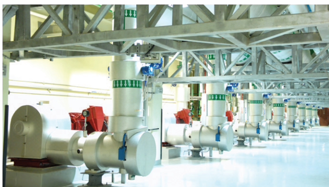
Photo 9: Primary chilled water pump installation with suction diffuser
