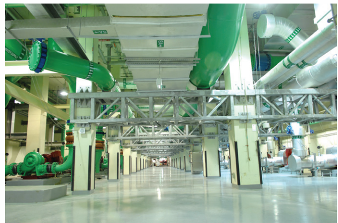
Photo 5: Pipe header supports in basement
