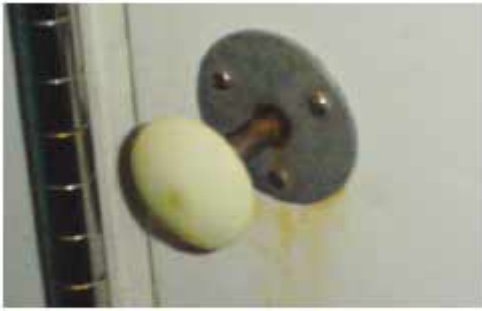
Safety release inside cold room which is photo luminescent, glows in the dark and provides an indication for the door opening lever.
