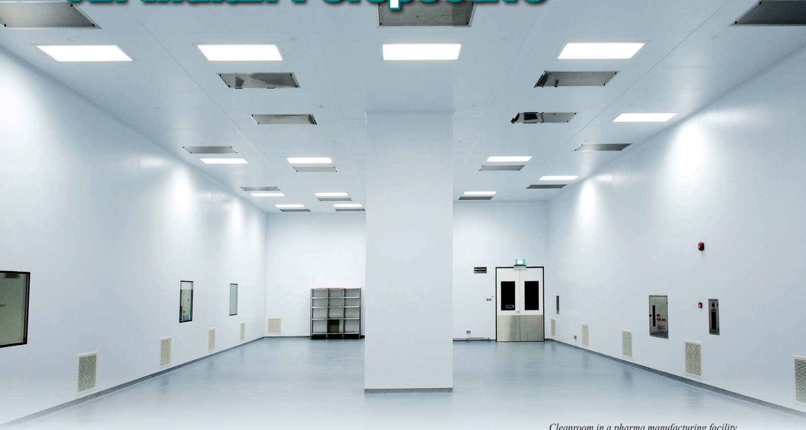
Cleanroom in a pharma manufacturing facility
