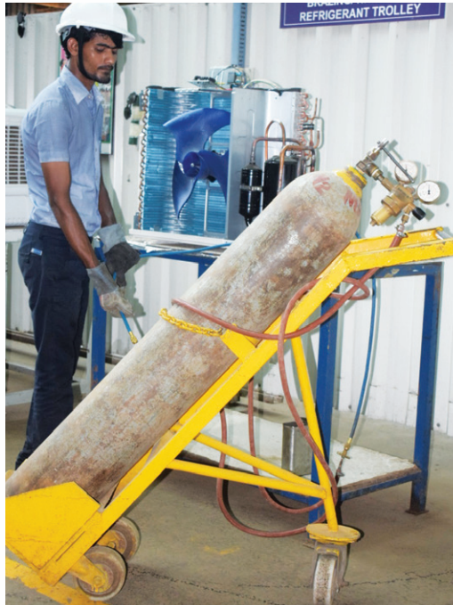
Figure 1: Nitrogen flushing before using cleaning agent to remove loose particles from system
