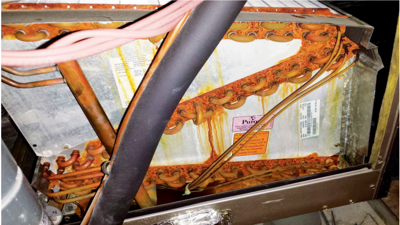
Formicary corrosion in a coil
