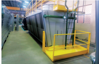
Figure 2: World's largest adiabatic cooler installation at Hindustan Zinc, Udaipur
