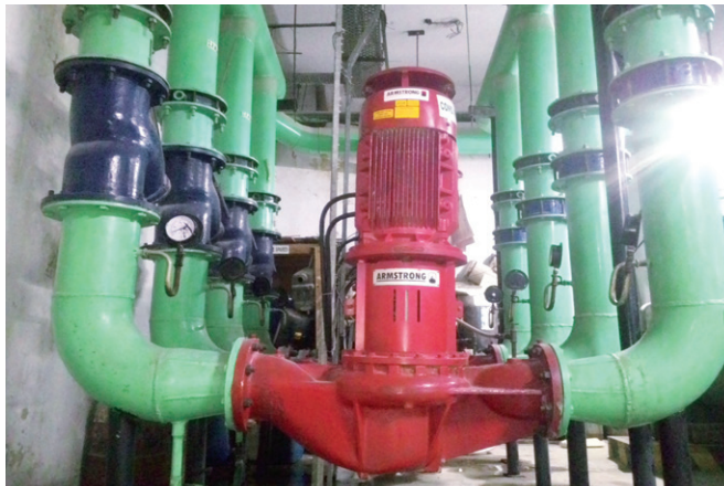
Photo 3: Inline condenser water pumps
