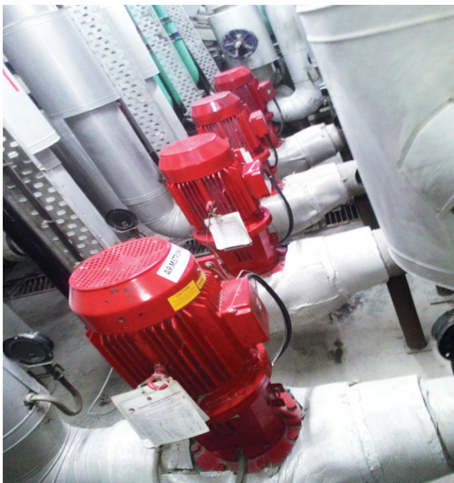
Photo 2: Inline chilled water pumps
