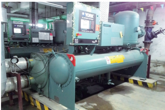
Photo 1: York chiller at PSRI
