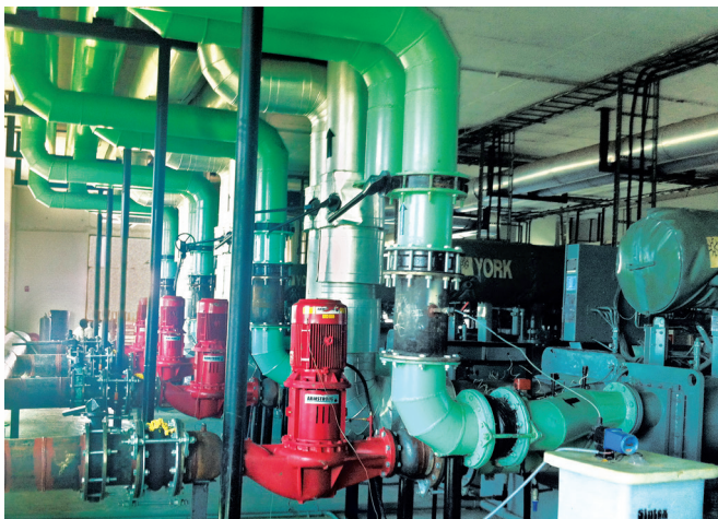
Figure 5: End-suction pumps – before retrofit
