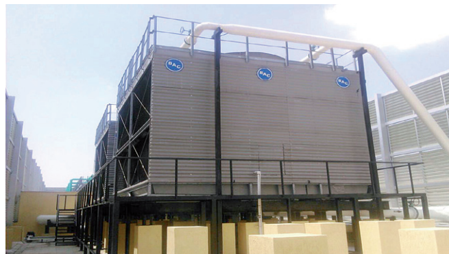
Photo 1: Cooling towers at the terrace
