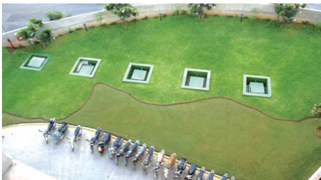
Photo 7 : Thermal Energy Storage Tank
