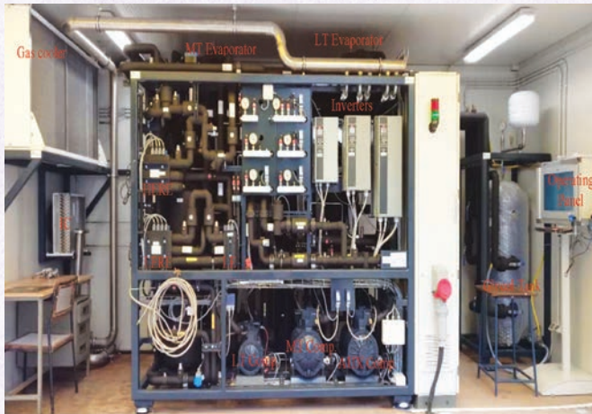
Figure 1: CO 2 cooling test facility
