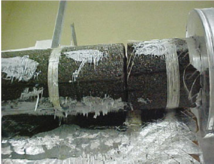
Photo 2 : Gap between adjacent pieces of insulation
