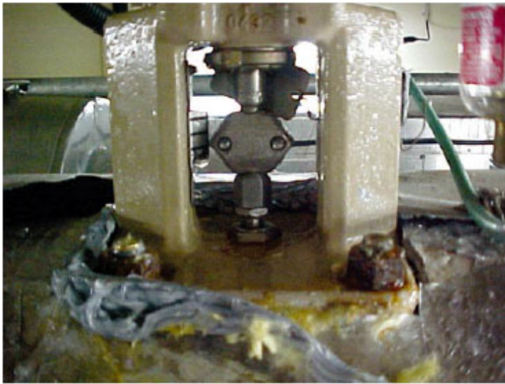
Photo 3 : Exposed valve stem without insulation
