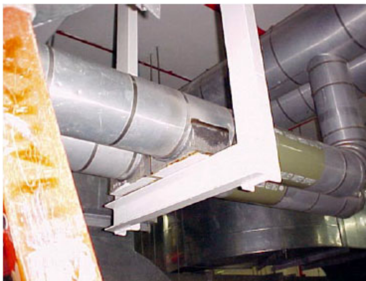
Photo 1 : Condensation on pipe support
