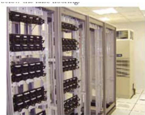
A Server room cooled by a standard packaged AC.
