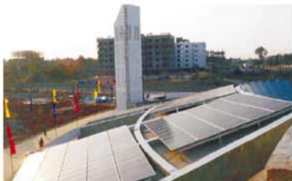
23kWp Solar PV system in GBC building.
