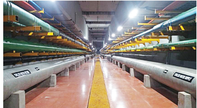
Figure 13: Chilled water pipe in utility tunnel
