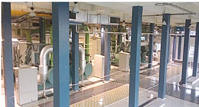
Figure 7: 10,000 TR chillers at DCP-1
