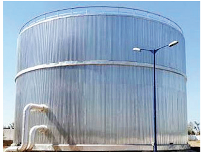
Figure 8: TES tank at DCP-1
