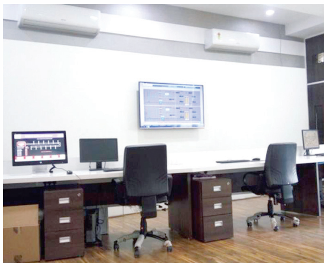
Figure 15: SCADA control room at DCP-1
