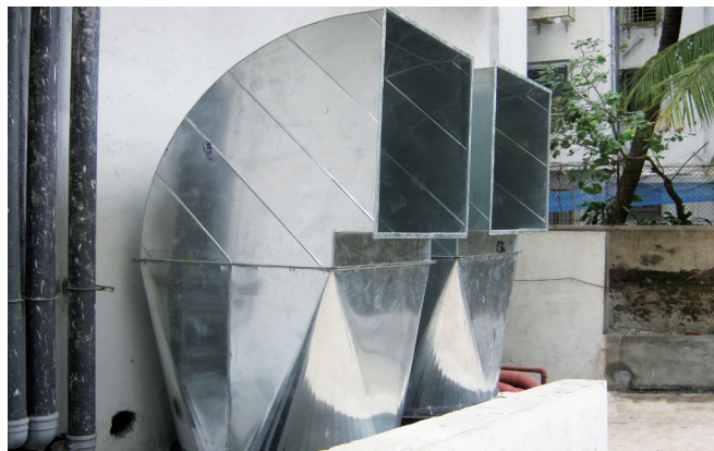
A basement exhaust outlet at ground level
