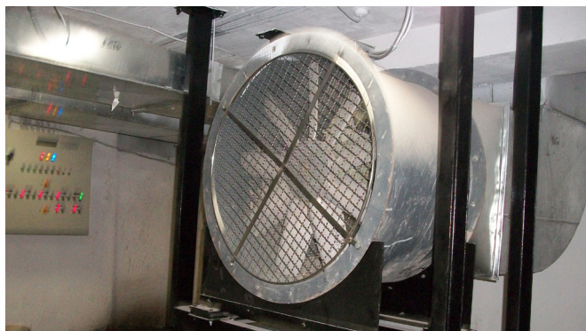
An axial flow fan at basement periphery
