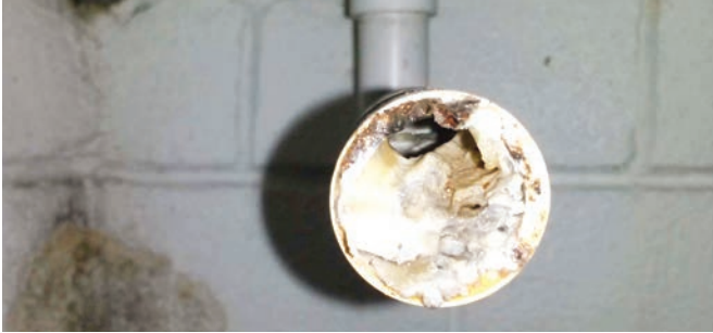
Figure 1: Contamination of drain
