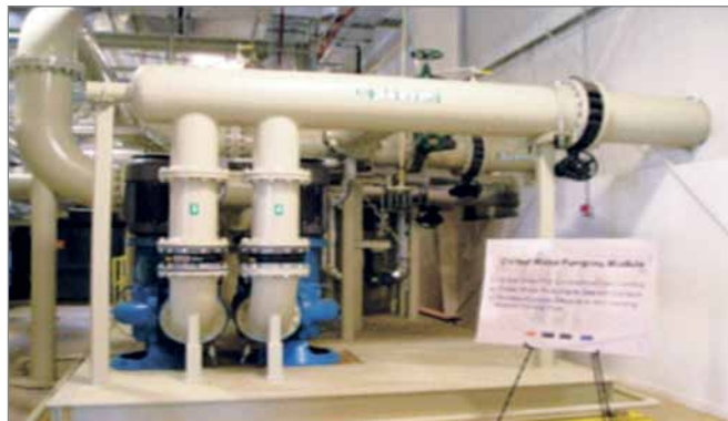
Photo 5: Chilled & cooling water pump station
