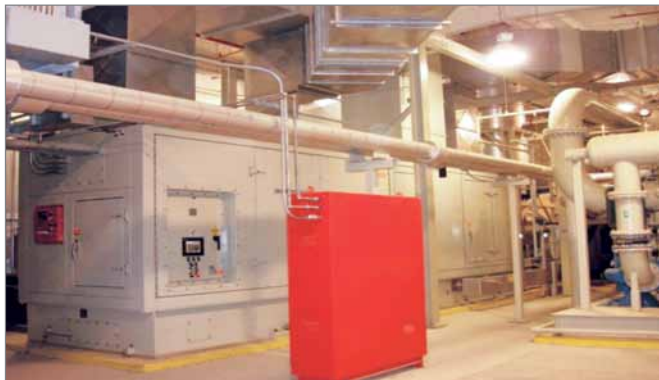
Photo 4: 5 MWe gas turbine package
