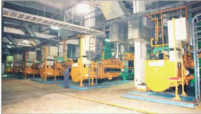
Photo 6: 7x1.4 MW gas engine generators
