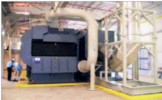
Photo 3: 2500TR heat recovery chiller coupled with a gas turbine
