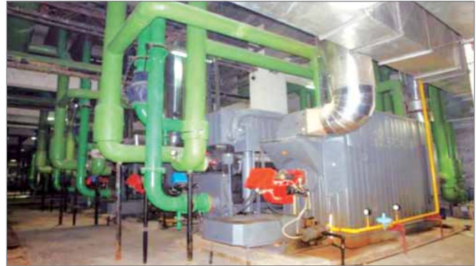
Photo 7: 7x500 TR heat recovery chillers
