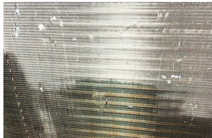
Photo 6: Restored coil area after deep cleaning and nano coating of fins (please note easy visibility of deep rows)
