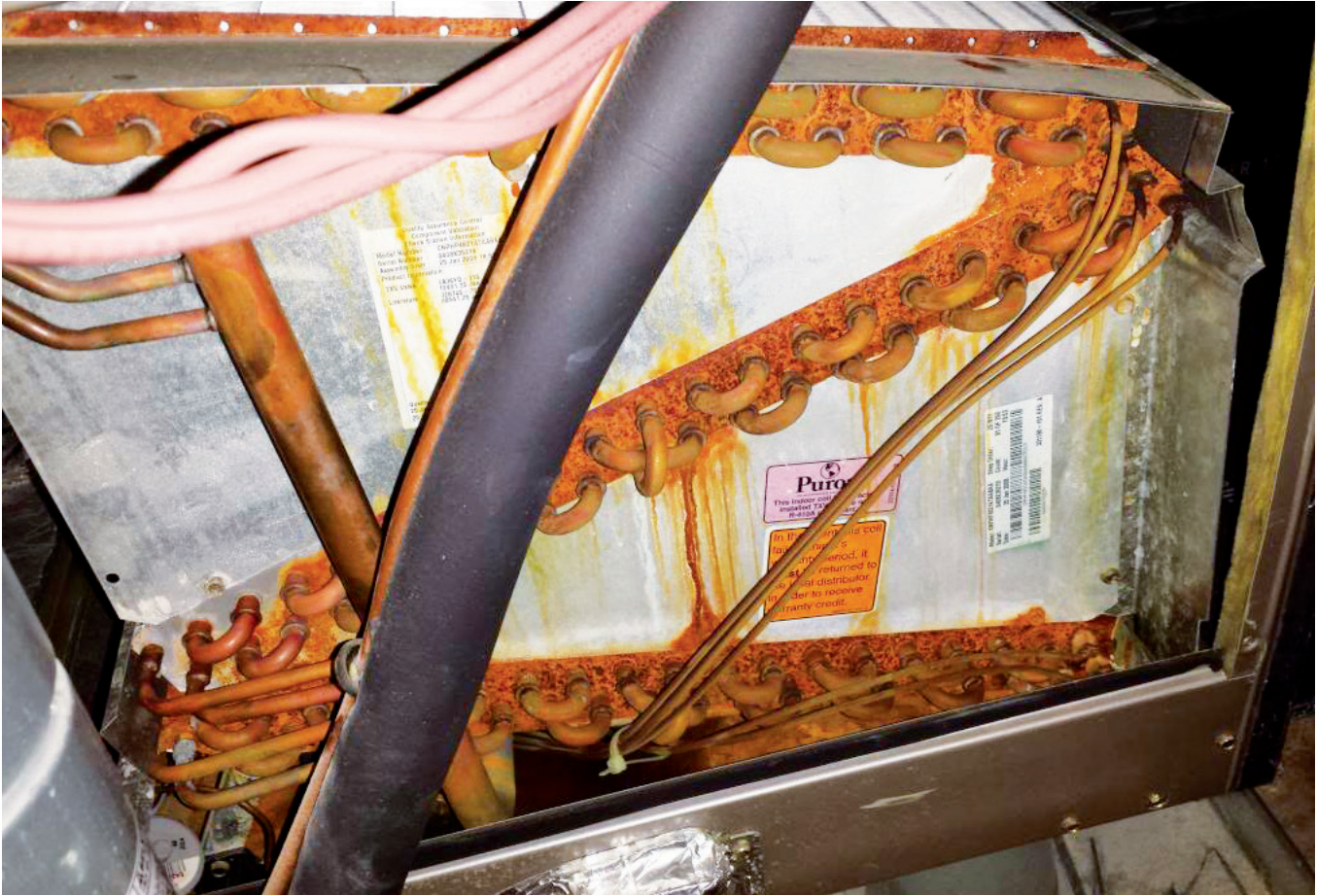
Formicary corrosion in a coil
