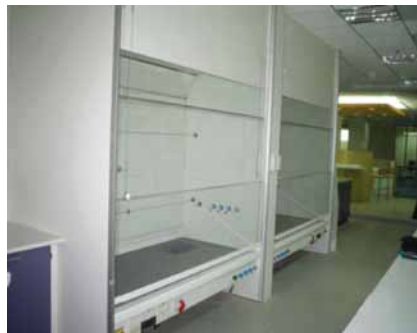
Photo 5 : Low level fume hood.
