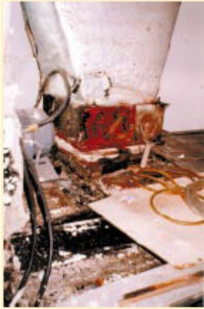
A view of the fan outlet damper, badly rusted and the flexible canvass connection with fungus growth.
