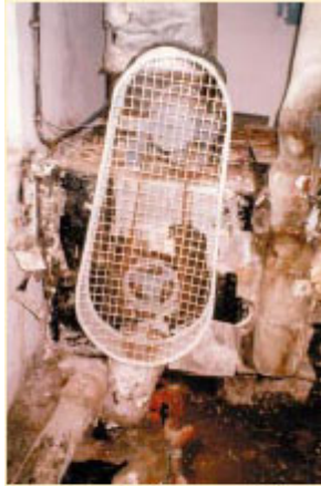
An end view of the AHU with external insulation
