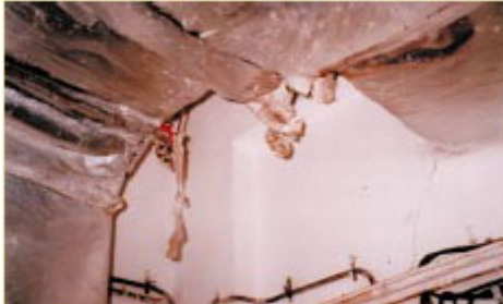
Aluminum vapor barrier separated from the duct insulation, and falling apart
