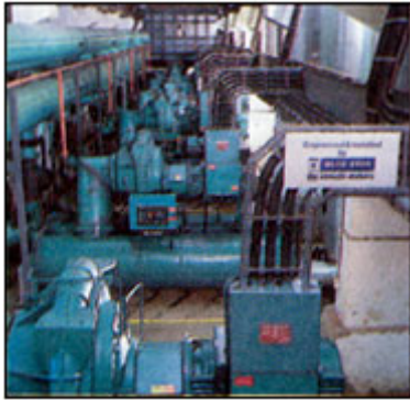
A central plant with centrifugal chillers
