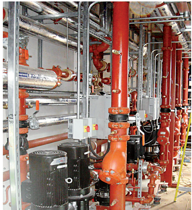
Installing a mechanical grooved piping system in London's Hackney Borough Council Customer Service Center reduced the total system weight and enhanced on site material handling
