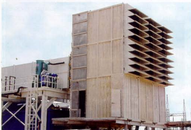
Photo 1: A typical inlet air evaporative cooling system
