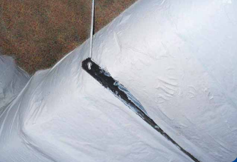
Weight of duct compressing insulation at duct support angle – a potential source of condensation
