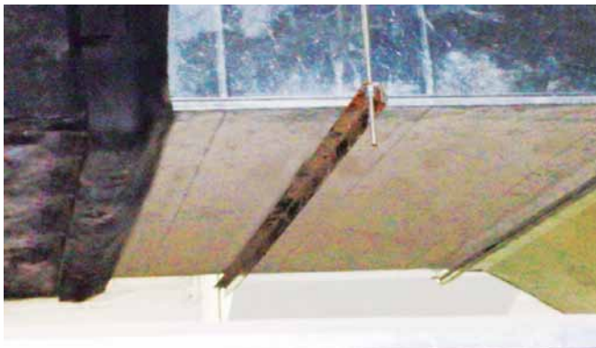
Photo 1: Condensation due to air gaps in fibreglass blanket insulation, leaking out of insulation joints
