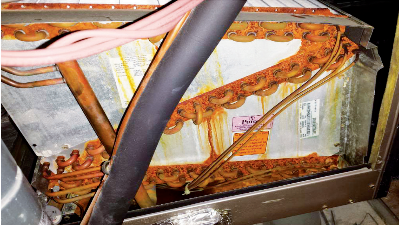
Formicary corrosion in a coil
