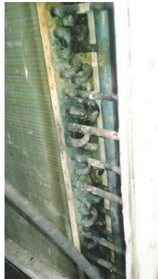
Figure 11: Old header with paint and rust oxides
