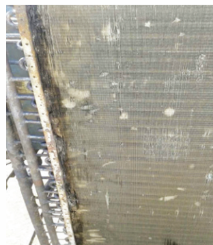
Figure 13: Old coil with dirt and corrosion
