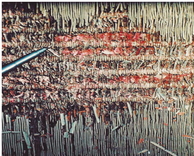
Figure 9: Copper coil exposed to salt air and burning of sugar fields, located 2 km from sea shore, for 18 months showing loss of fins and built-up oxides
