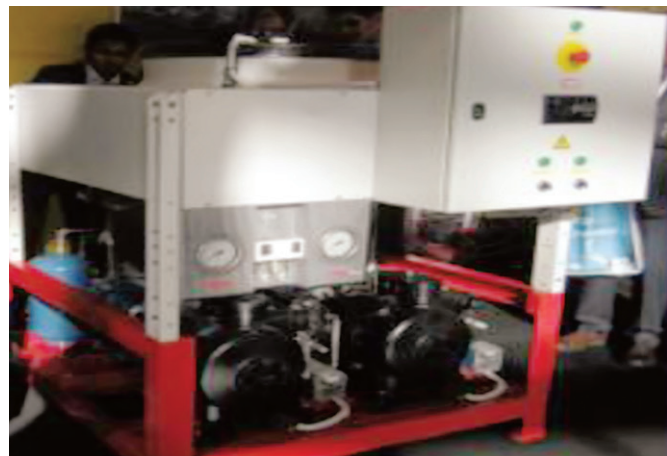
Photo 14: Ammonia reciprocating compressor package
