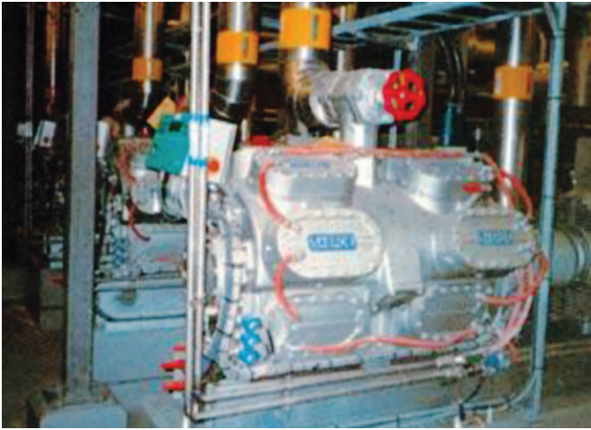
Photo 1: Plant room at Oslo airport
