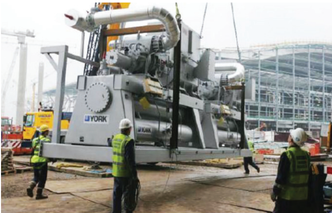
Photo 2: One of the four package ammonia chillers being installed at Heathrow airport
