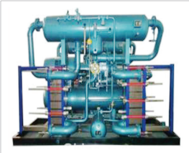
Photo 16: Ammonia packaged chiller
