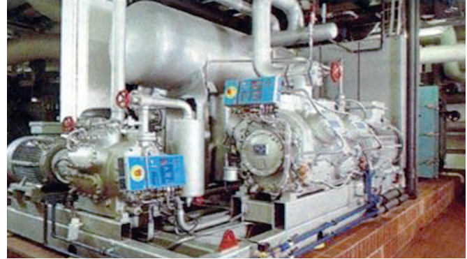
Photo 4: Ammonia chiller package at P&T Building, Copenhagen
