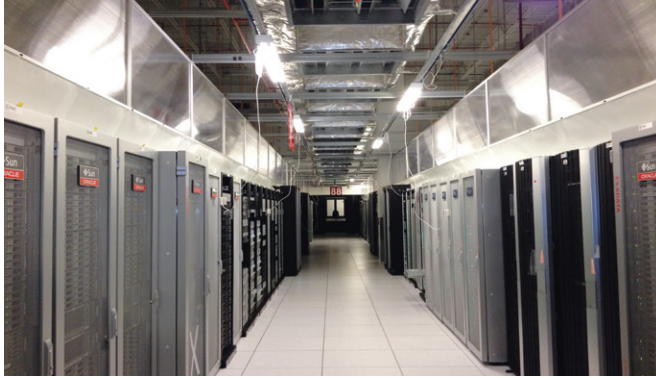
Cold aisle showing partial un-containment at the data center.
