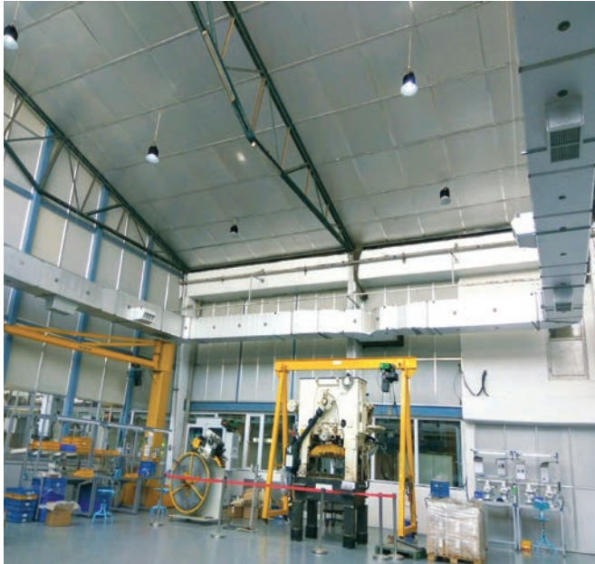
Photo 1: Installation with underdeck insulation with ducting running in the conditioned area
