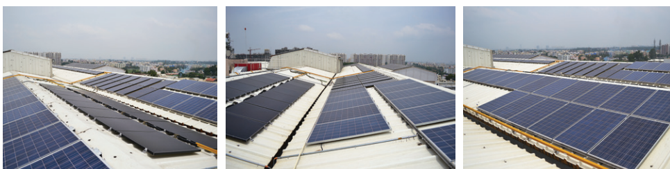
Figure 6: Different solar PV technologies on the roof of EC-53 building
