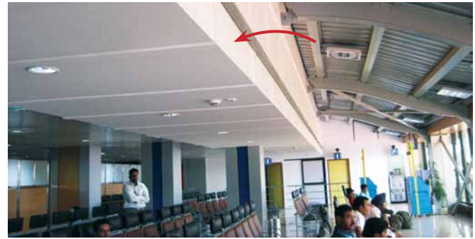
RA duct at the Pune Airport made of fire resistant material. Photo courtesy : Promat International.
