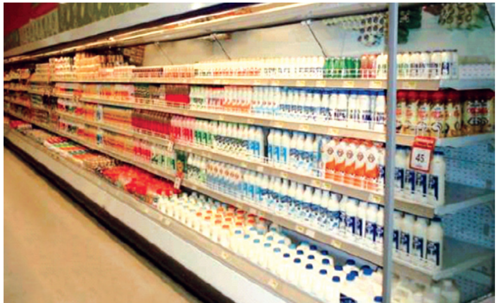
Photo 3: Display cases with remote compressor unit.
