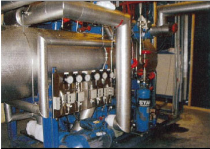
The demonstration unit: the compressor drive motor (55 kW) is in the foreground
