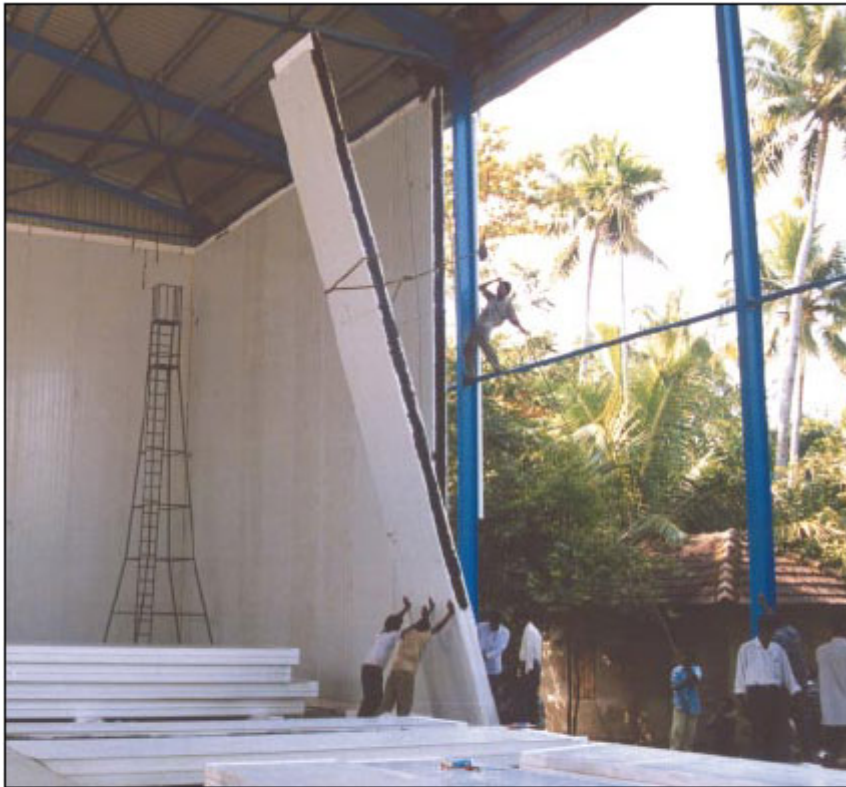
Photo 1 : A large cold store with pre-fab insulated panels under installation for Snowman Frozen Food, Kochi. Room dimensions 50 × 20 × 9.5m high. Photo courtesy of Beardsell Ltd.
