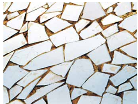
Photo 5 : Broken china mosaic tiles on roof.
