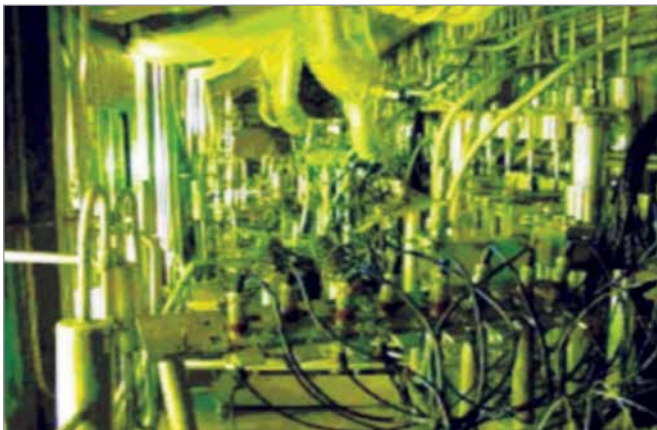
Hot cell for reprocessing of spent fuel: Typical red zone
