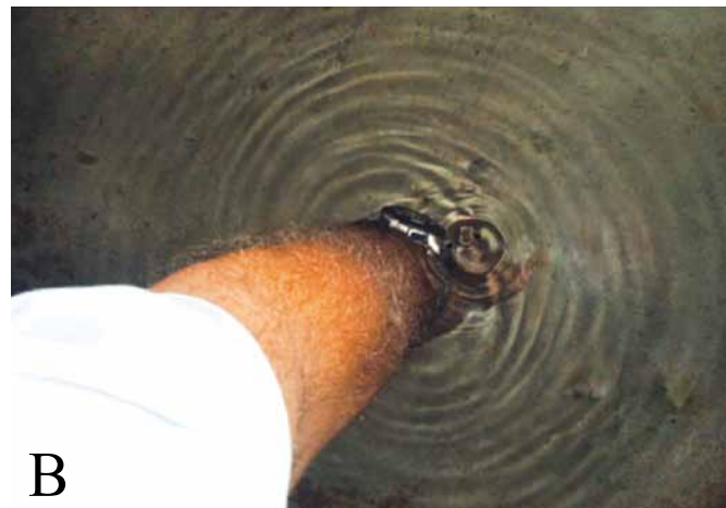
Photos 1a and 1b: Condensate pan overflow into return air plenum caused by blockage of condensate drain line.
