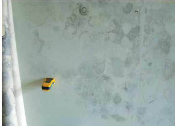
Photo 3: Mold growth in a wall cavity depressurized by a return plenum. 2
