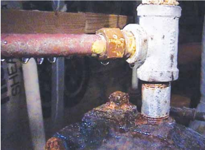
Photo 2: Condensation on an uninsulated chilled water line in an unconditioned space. 2
