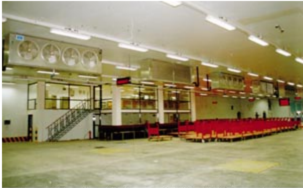
An inside view of the new Perishable Cargo Centre with Bohn product coolers installed in the middle of the Pre-staging area.
