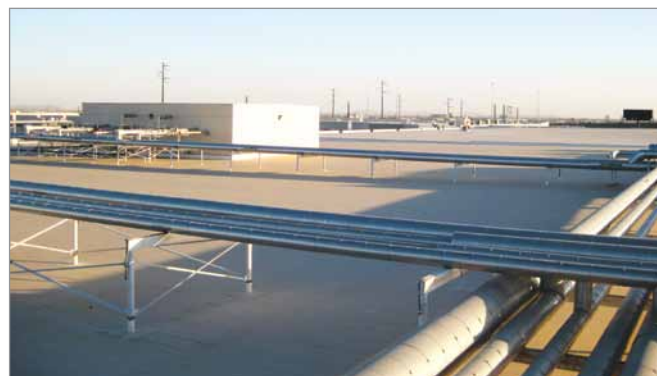
Photo 13 : Outside view of the cooling unit room or 'dog-house'
