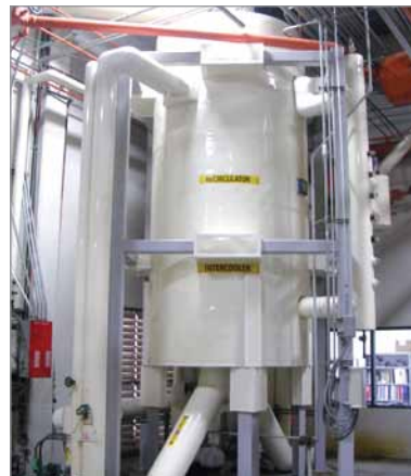
Photo 15 : Another view inside the plant room
