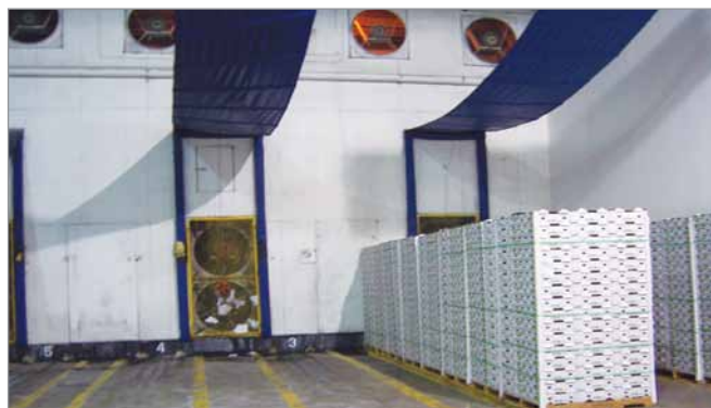
Photo 5 : Inside view of the pre-cooling rooms with pallets loaded for one cooler
