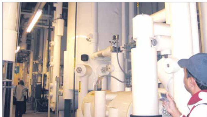
Photo 14 : Inside view of a plant room
