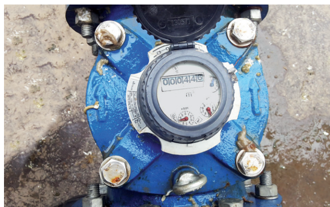
Figure 7: Water meter to monitor condensate flow rate
