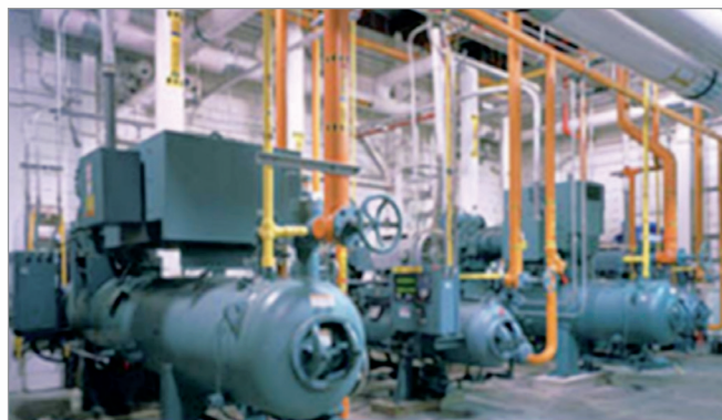
Figure 10: Typical energy efficient two stage compound compressor
