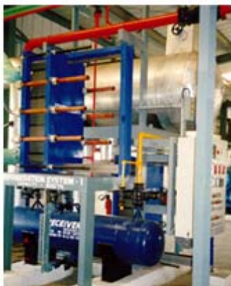
General view of a 200 ton Ammonia refrigeration plant. Photo courtesy of the author.
