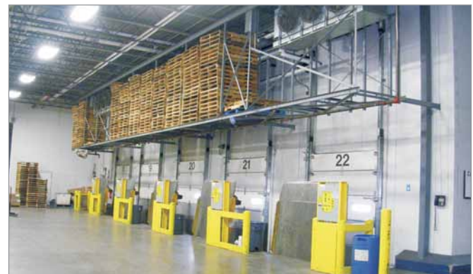
Photo24 : Dock doors from the inside. Notice that the dock levellers are kept fully upright
