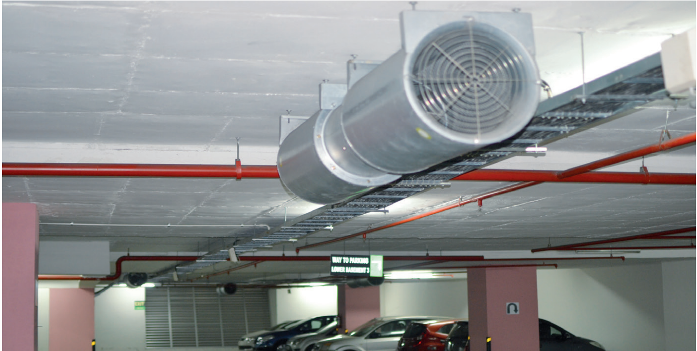
A jet fan installed in an enclosed car park
