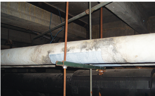
Photo 4: Major water damage.
