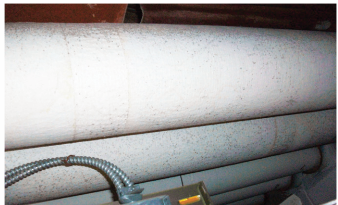
Photo 6: Mold spotting caused by excessive humidity.
