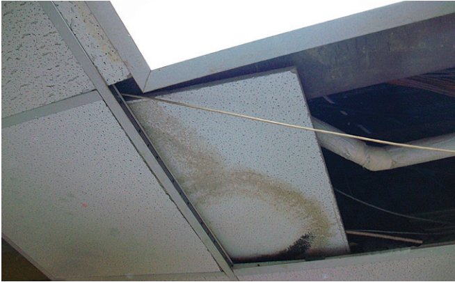
Photo 3: Stained ceiling tile under sweating chilled water pipe.
