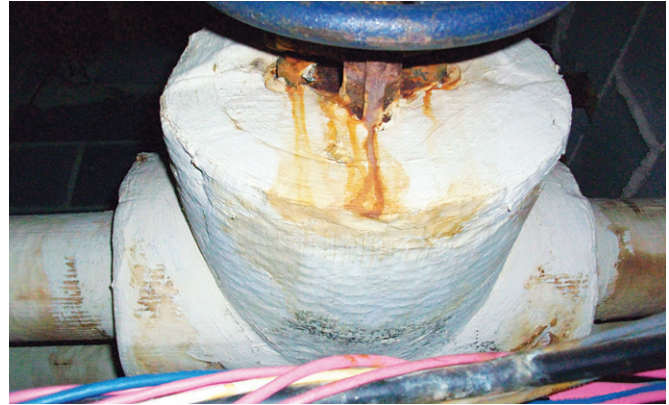
Photo 5: Minor water damage.
