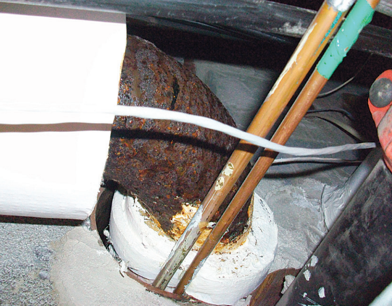
Photo 1: Pipe section left unsealed.
