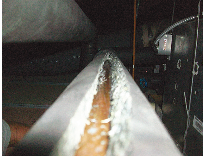
Photo 2: Insulator failed to seal top seam.
