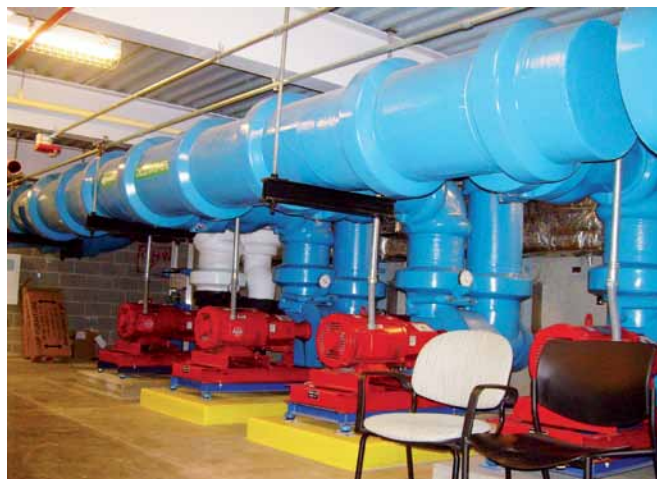
Photo 3: Primary chilled water pumps & header
