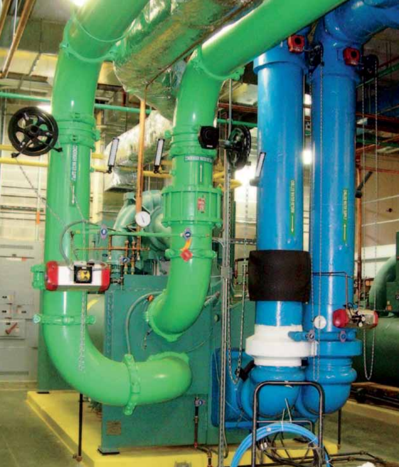
Centrifugal chiller installed in the Central Plant room
