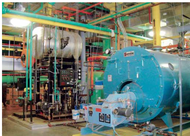
Photo 2: Boilers installed in the Central Plant Room
