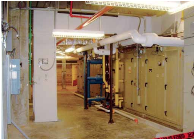
Photo 1: Typical custom built AHU
