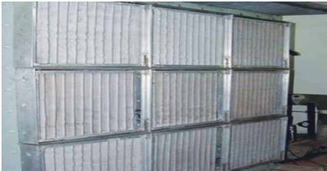
Figure 2: View of retro fitted new high performance aluminium extruded Universal Holding Filter Frames (UHFF).
