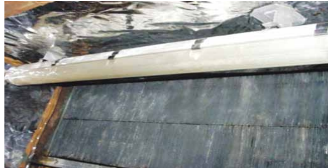
Figure 5: View of UVC (Ultra Violet C Band) germicidal lamp, fitted inside the AHU-5
